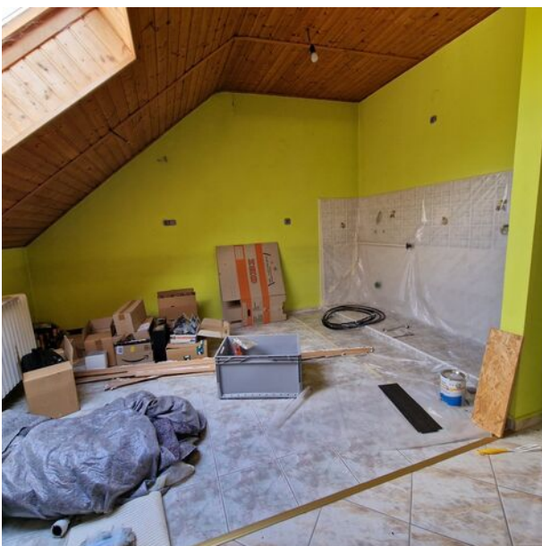
Kitchen prepared above
