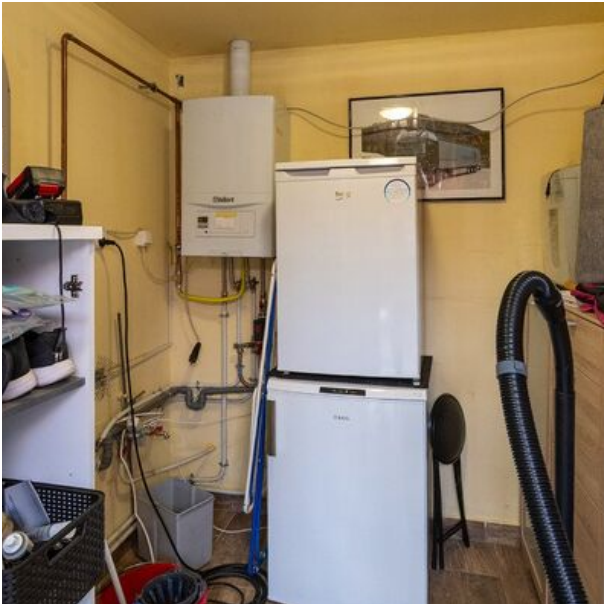
Technical utility room with modern heating system and practical storage facilities
