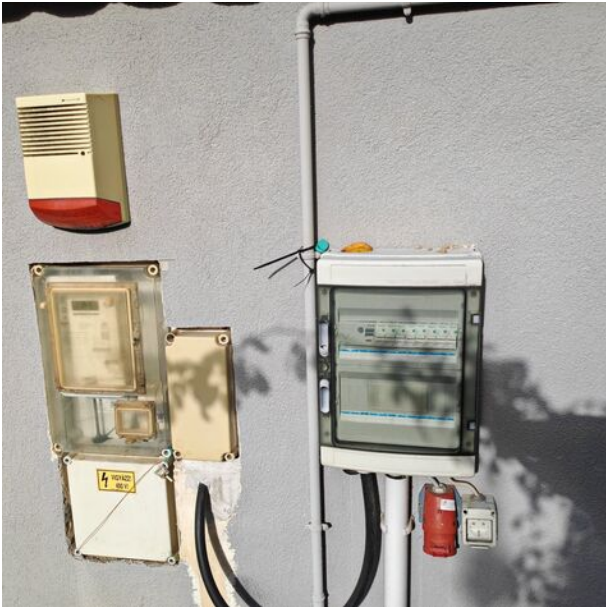
Latest electrical system
